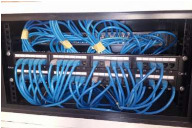
Figure 6: Patch panel and Cables
